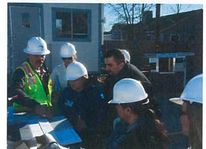
CBOC Committee Members working with Contractor on final finishes for the Arbuckle Elementary School's New
